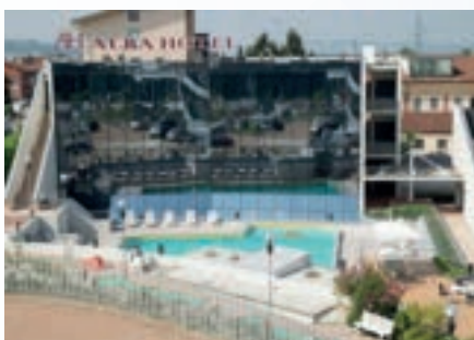
FOE HOTEL ALBA in Italy Hot water / 135RT 1 unit
